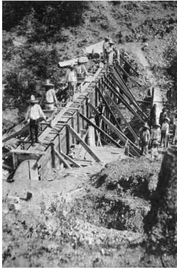
PLATE V, FIG. 2.—PLACING CONCRETE PIPES IN FORMS FOR BRIDGE CROSSING AT NORTH END OF TUNNEL, ESTANZUELA AQUEDUCT.
