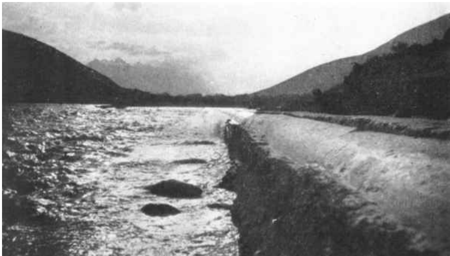
PLATE XXXI, FIG. 2.—VIEW SHOWING SCOURING EFFECT OF FLOOD ON SAN GERONIMO AQUEDUCT.
