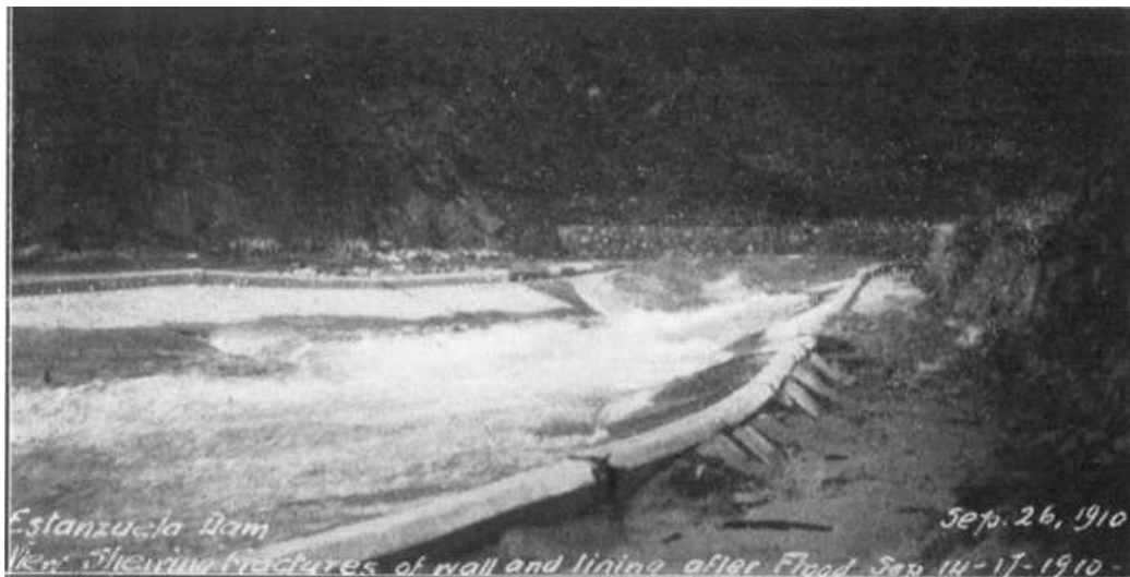
PLATE XXXIII, FIG. 3.—ESTANZUELA DAM SEPT. 26, 1910: VIEW OF SHEARING FRACTURES OF WALL AND LINING AFTER FLOOD SEPT. 14-17, 1910.
