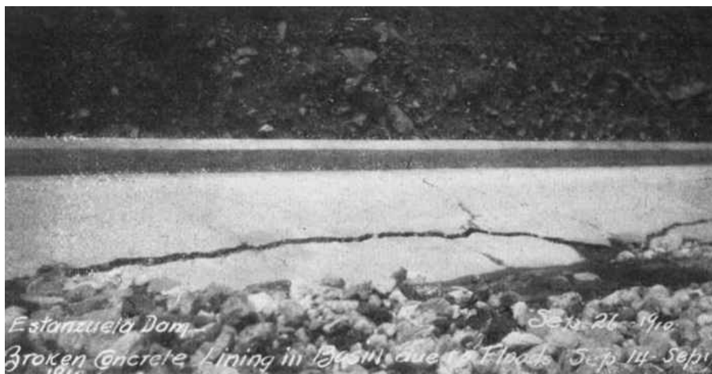
PLATE XXXIII, FIG. 1.—ESTANZUELA DAM: BROKEN CONCRETE BASIN LINING.
