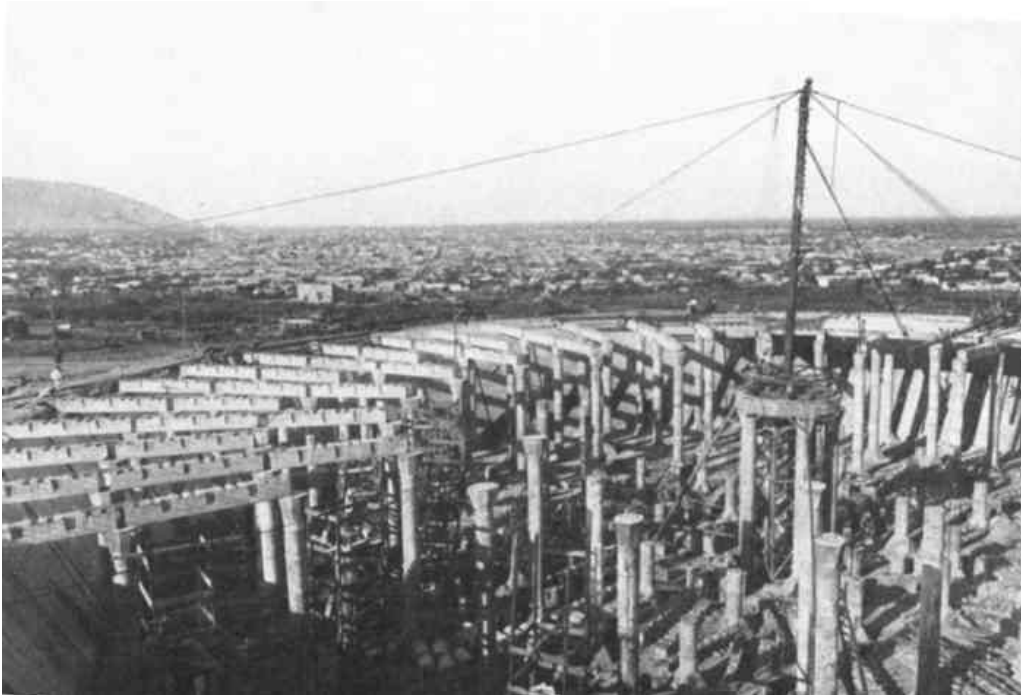
PLATE VIII, FIG. 2.—VIEW OF WESTERN HALF OF SOUTH RESERVOIR, SHOWING FINAL SETTING UP OF DERRICK ON CENTRAL COLUMNS.
