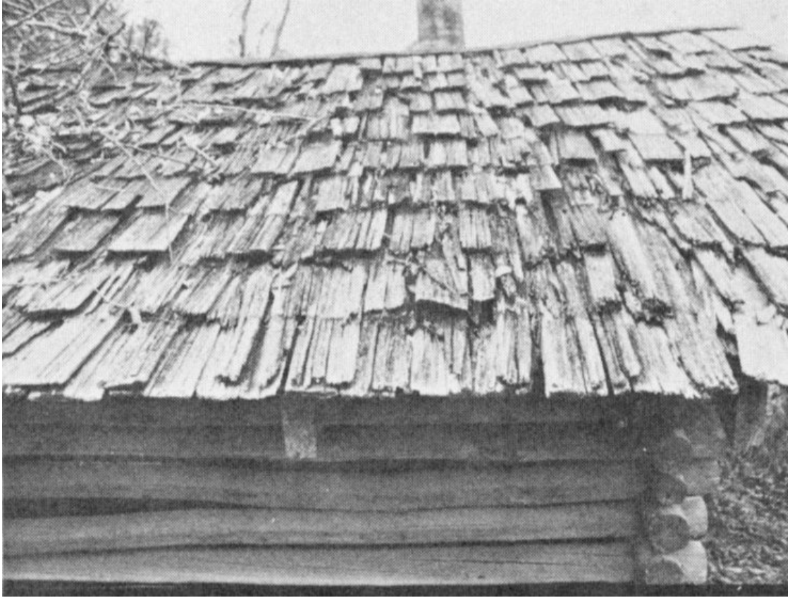
18. Shingle or board roof. Tool shed, Walthall County. Present owner: George Wingo
