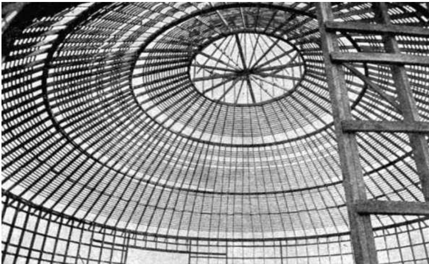
FIG. 35. VIEW OF 70-FOOT SELF-SUPPORTING ROOF ON BARN SHOWN IN FIG. 36 ; NOTE HOOPS ON STUDS IN RIGHT FOREGROUND.
