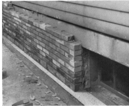
Start of Veneering over Frame Note footing below and wall ties above
