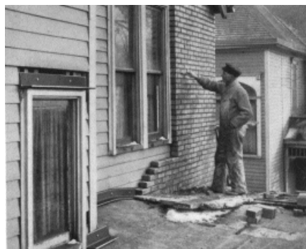
Veneering above Kitchen Roof Note angle irons and work at windows
