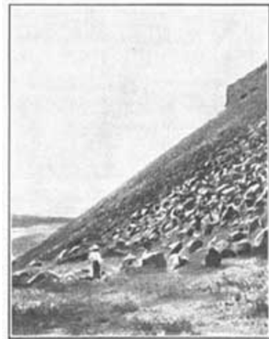
FIG. 21.—The destruction caused by freezing water.
